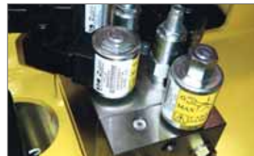
Hydraulic system line assembled, improves security and full power on cylinders.
