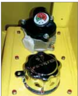
Oil level control
